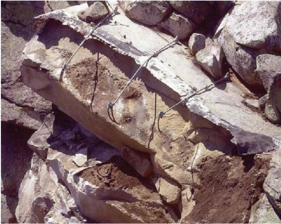
Figure 9. Close-up, top of the Profile's residual rock mass (photo by Union Leader Corp., 2003).
